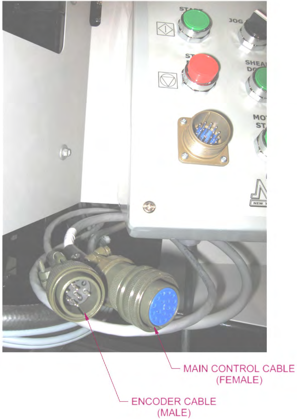
Figure 2: Main Control Cable
